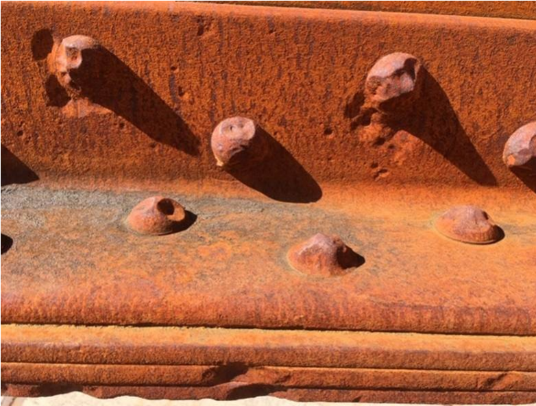
Fig. 7. Corroded rivets in bottom flange.
